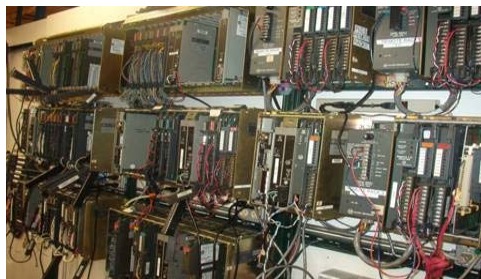
ALLEN BRADLEY PLC'S
